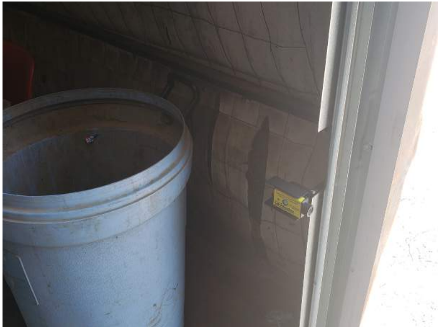
Torn insulation fabric
