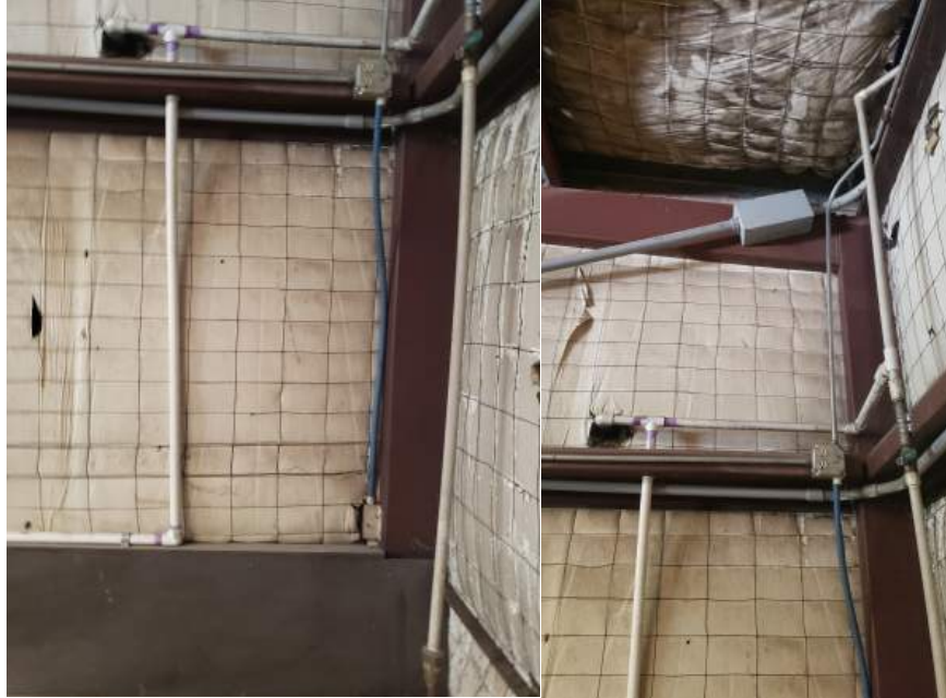
Tears and staining of insulation
