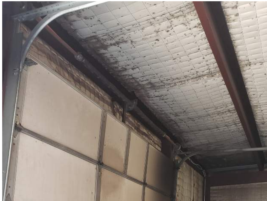
Moisture damage and mold on insulation
