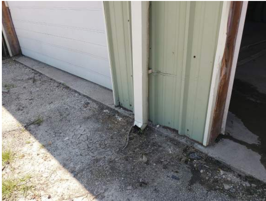
Impact damage on door frame and siding
