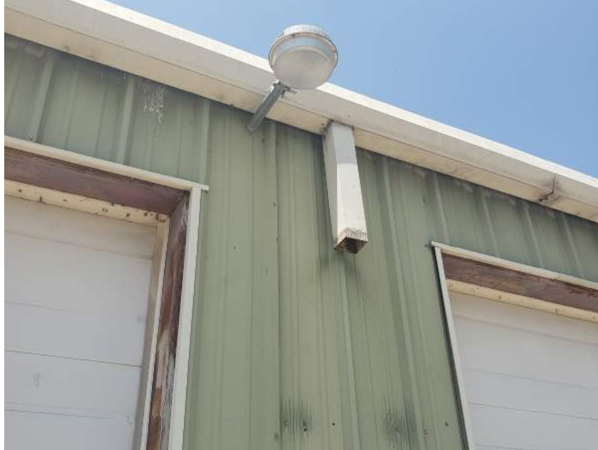
Disconnected downspout, moisture damage at gutter seams
