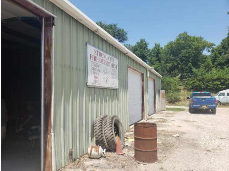
Faded exterior, impact damage, rusting door frames
