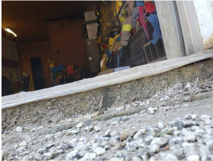
Degrading site earthwork and non-ADA compliant entry
