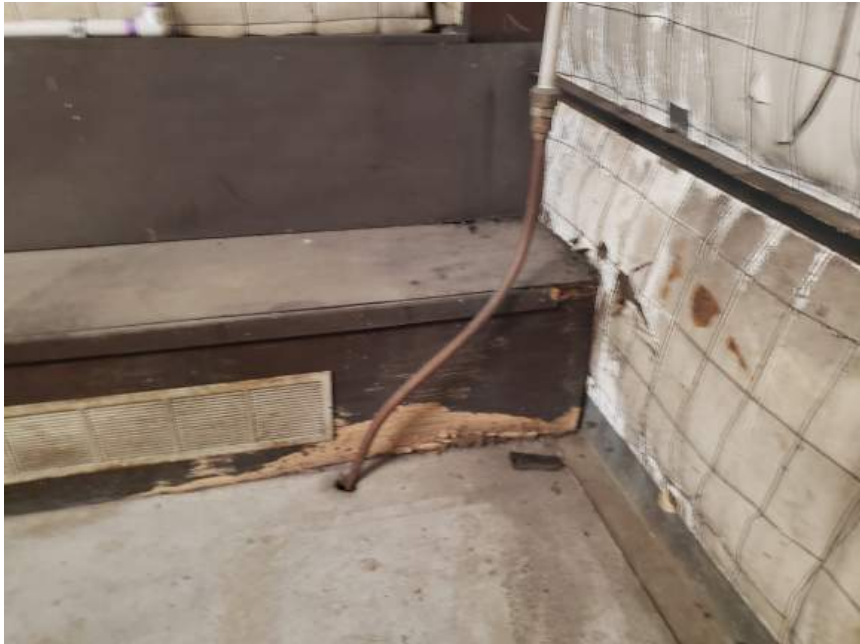
Deterioration of HVAC chase
